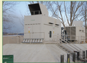
CNG Fueling Station
