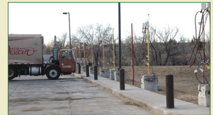
Fuel Lines for Fueling CNG Trucks
